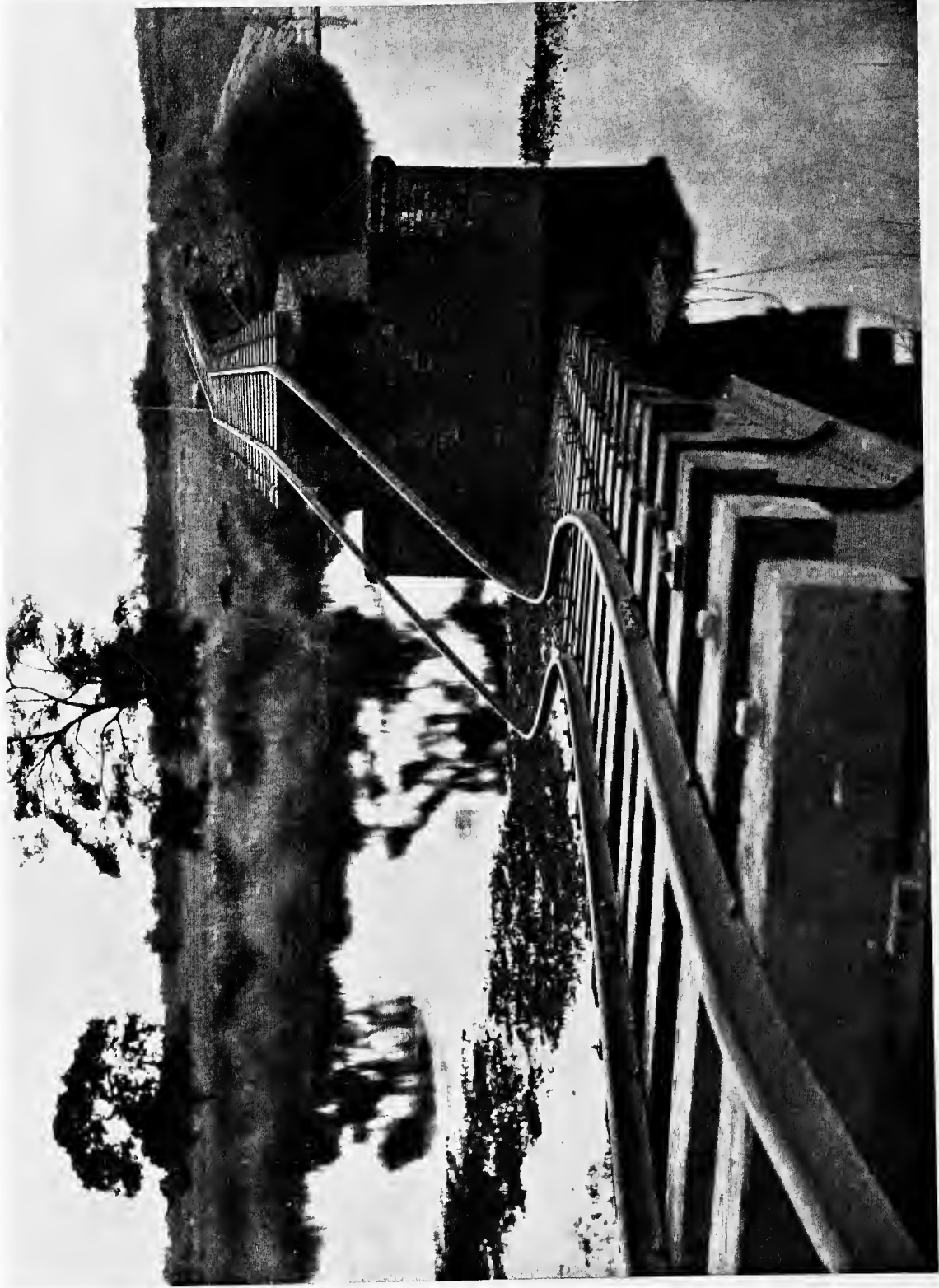
AFTER THE EARTHQUAKE : ON THE COOCH BEHAR STATE RAILWAY.
